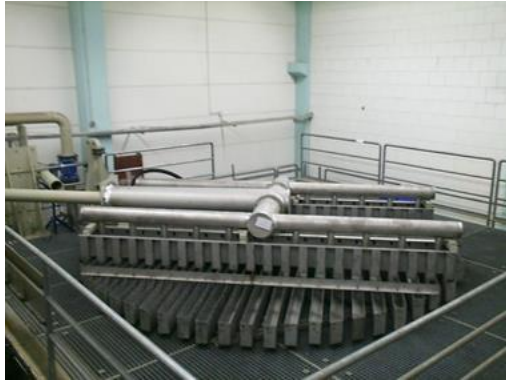
Test bed equipped with trough type distributor P114_RVT_TestFacilities_pic4
